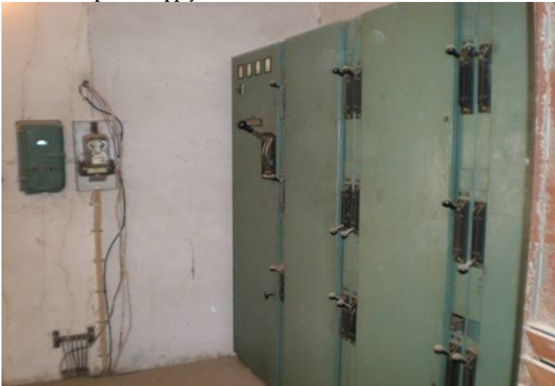
ii. Picture of power Supply Panel.
